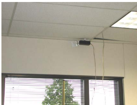
Figure 2. Another typical ceiling mount for PAL-650 Receiver.
