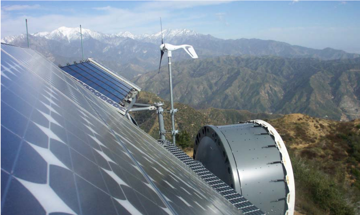
Figure 30 Example of Solar and Wind Power Installation
