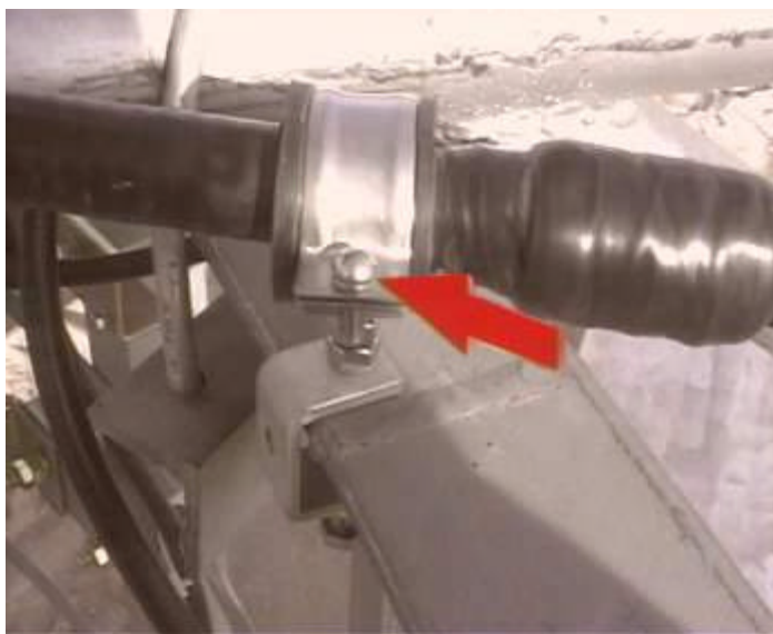
Figure 3-35 Feeder upper end fixed on tower
