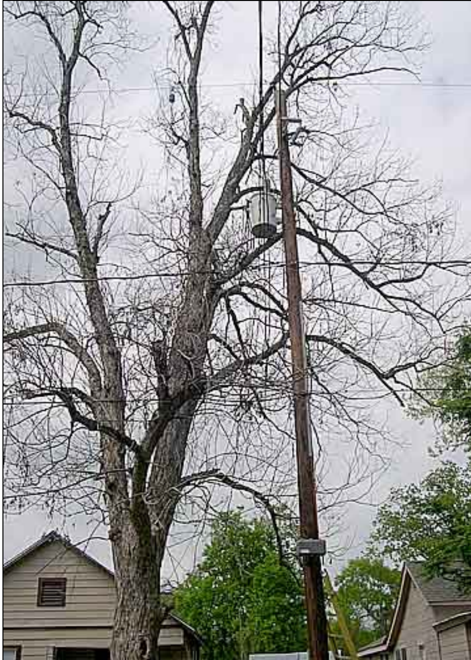
EUT Installed on Pole
