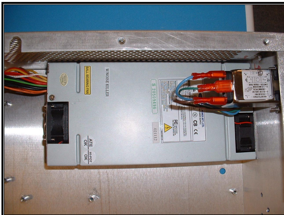
PHOTOGRAPH 18: AC LINE FILTER IMPLEMENTATION #4
