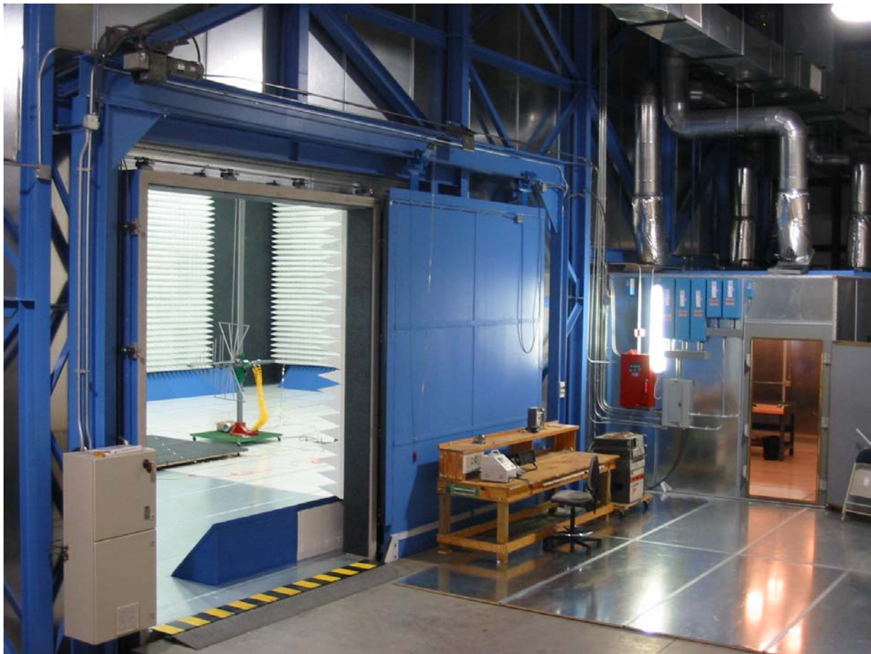
Figure 3-1: 10-Meter EMC Site
