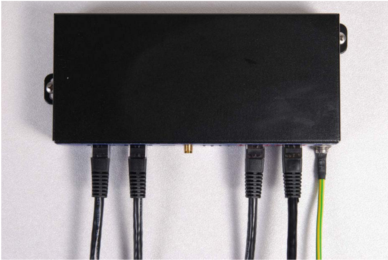
Figure 113 PTP-SYNC mounted on a wall
