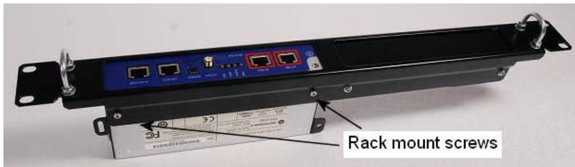
Figure 112 PTP-SYNC mounted in a rack
