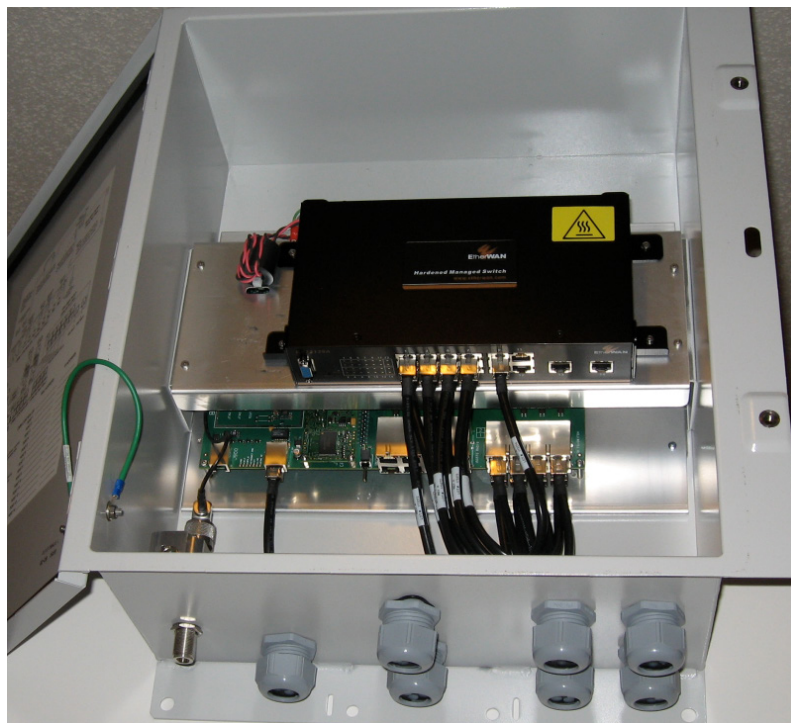
Figure 40 CMM4 (Cabinet with switch)
