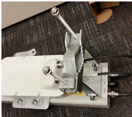
Figure 87 Lower bracket attached to AP antenna
