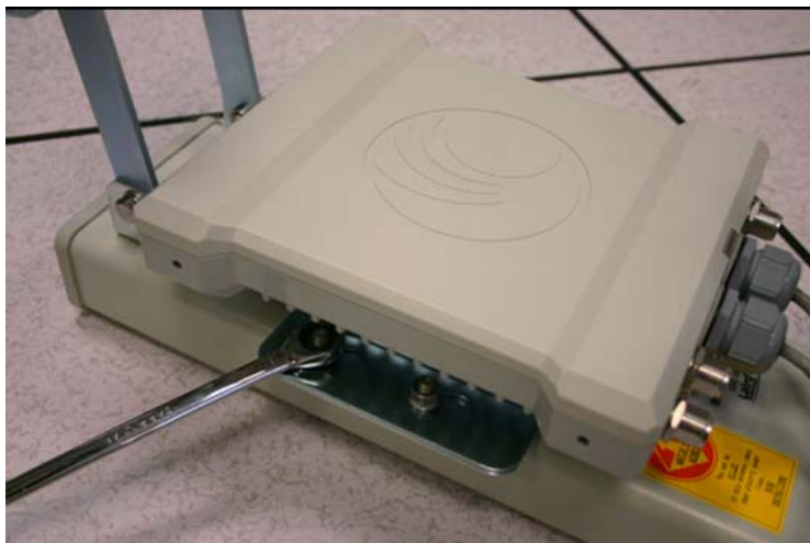
Figure 97 Lower bracket attached to AP antenna
