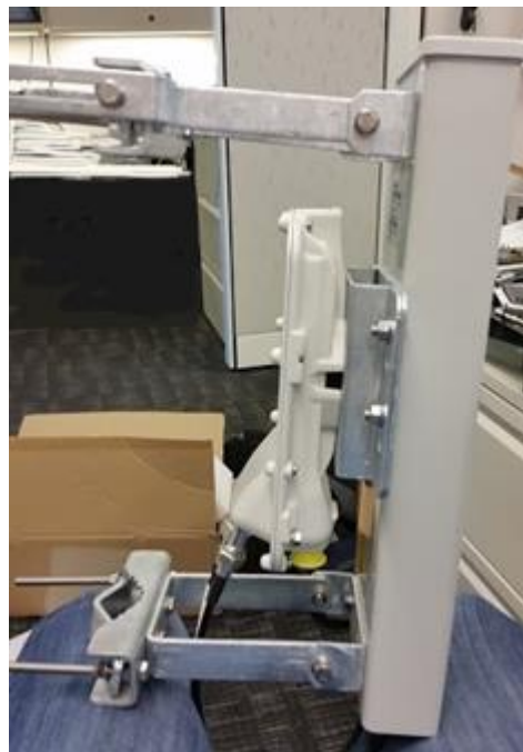
Figure 67 Completed AP and antenna assembly
