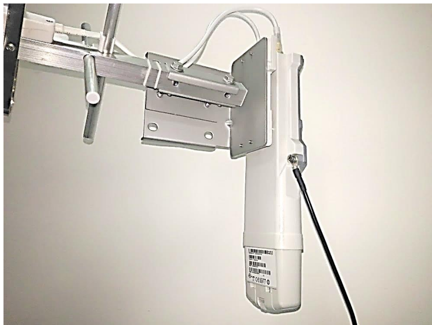
Figure 48 PMP 450 900 MHz SM grounding
