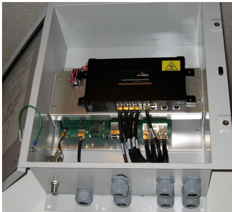
Figure 33 CMM4 (Cabinet with switch)
