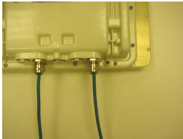
Figure 11 - Making the Network Connection
