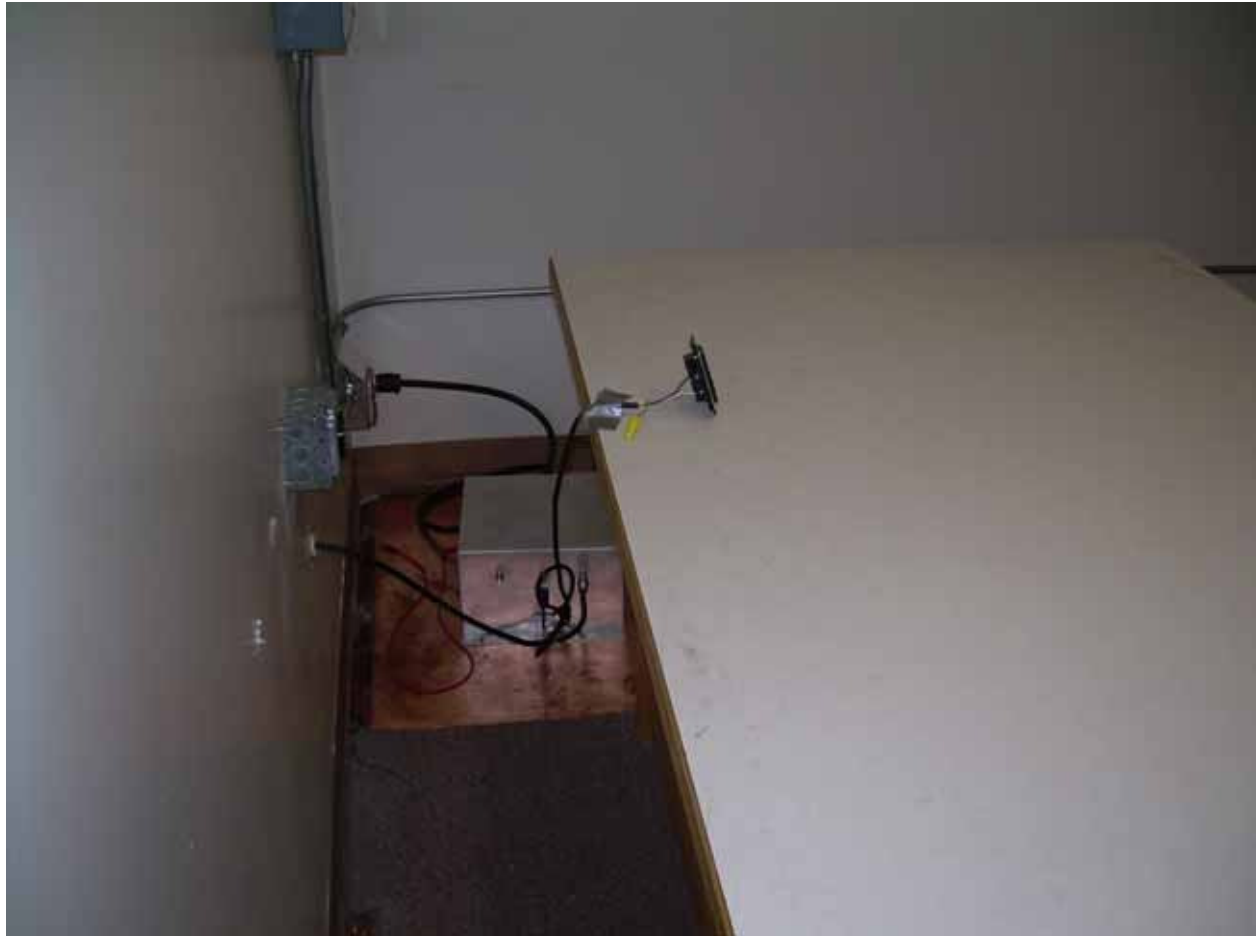
Photograph 4 – Back View Conducted Disturbance Worst Case Configuration
