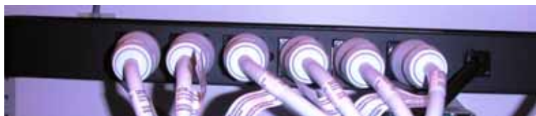
Figure 20 - Electrical Connections in the Powered Auxiliary Cabinet
