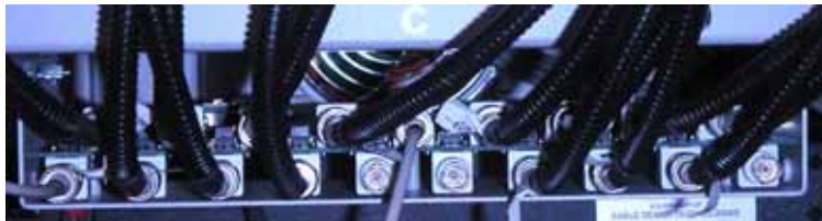
Figure 14 - Antenna Cable to Multiplexer Connection
