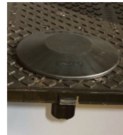
Figure 2.26 Antenna hole in pit lid
