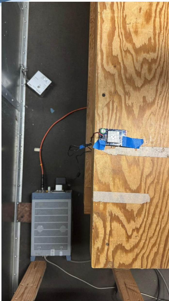
AC Wireline Setup (Side)
