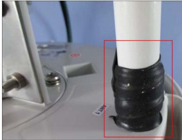
Figure 28 Layer of rubber insulation on antenna connection
