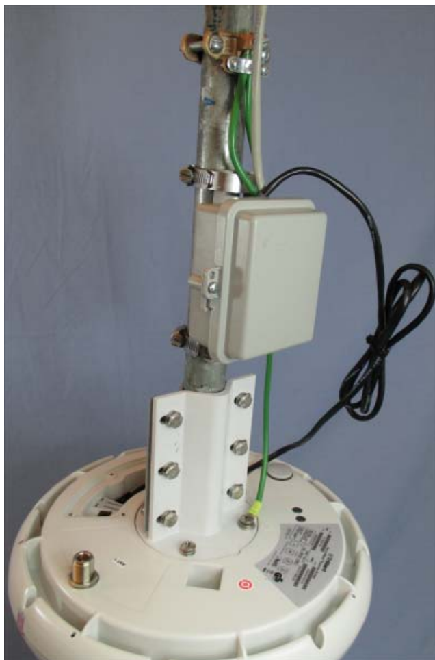
Figure 11 Assembled and mounted Citel surge protector
