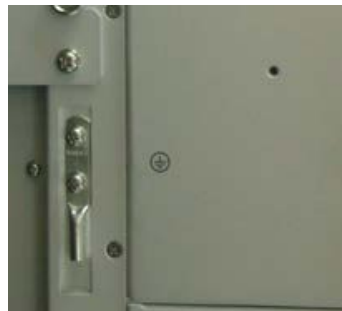
Figure 4-2 Ground Cable Connection
