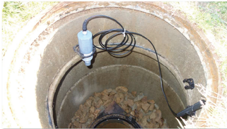
Positioning of a Sigfox antenna 1
