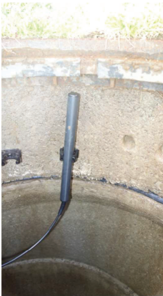
Positioning of a Sigfox antenna
