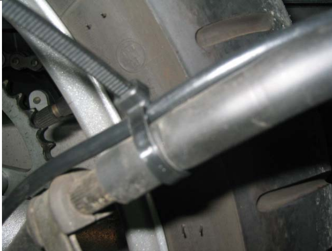
Fig. 10 Tie-wrap loose wires
