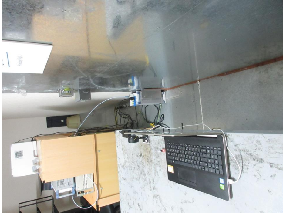
Photograph 9: Set-up for AC Mains (Back View)
