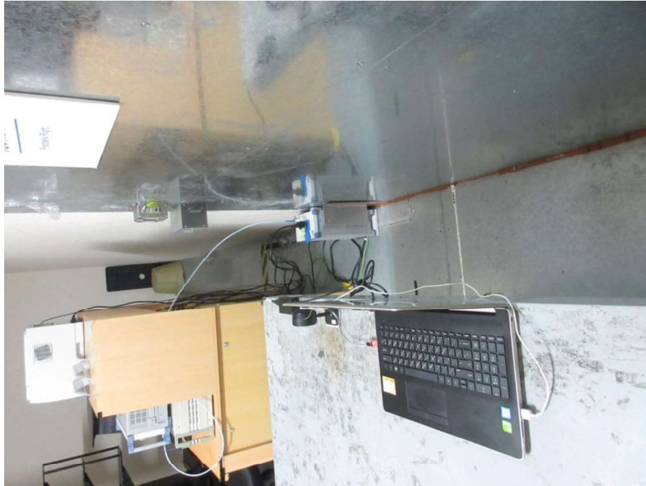
Photograph 9: Set-up for AC Mains (Back View)
