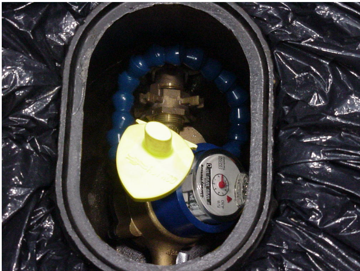
Figure 2 – Photo of EUT Installed in Meter
