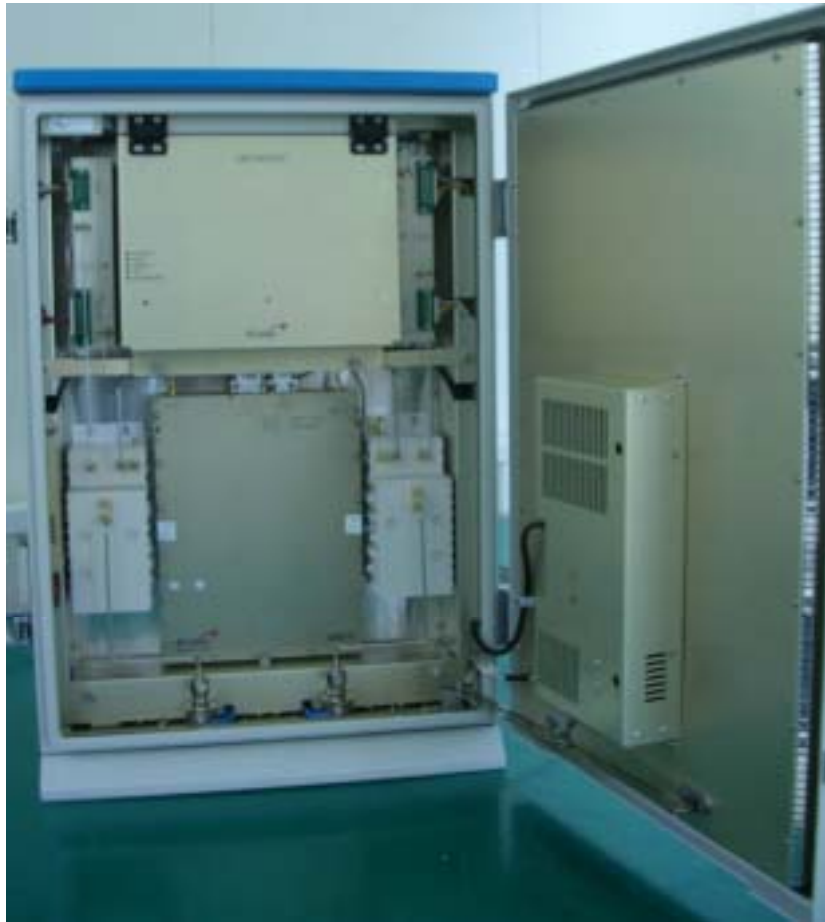
< The Inside of the Repeater >
