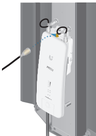
Connecting the GPS Antenna
