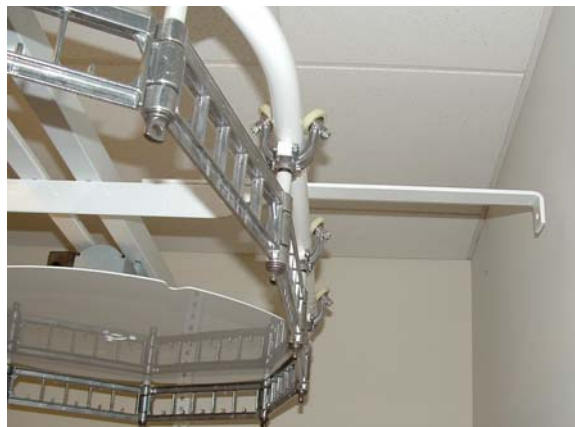
Example: View of rear sway brace for machine. Should be positioned against the wall and secured with a lag screw.
