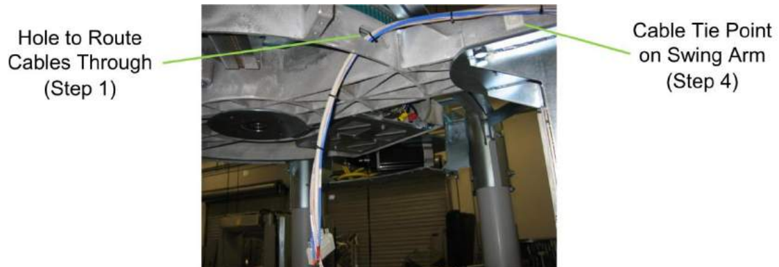
Figure 55: Cables Routed Through Swing Arm Hole
