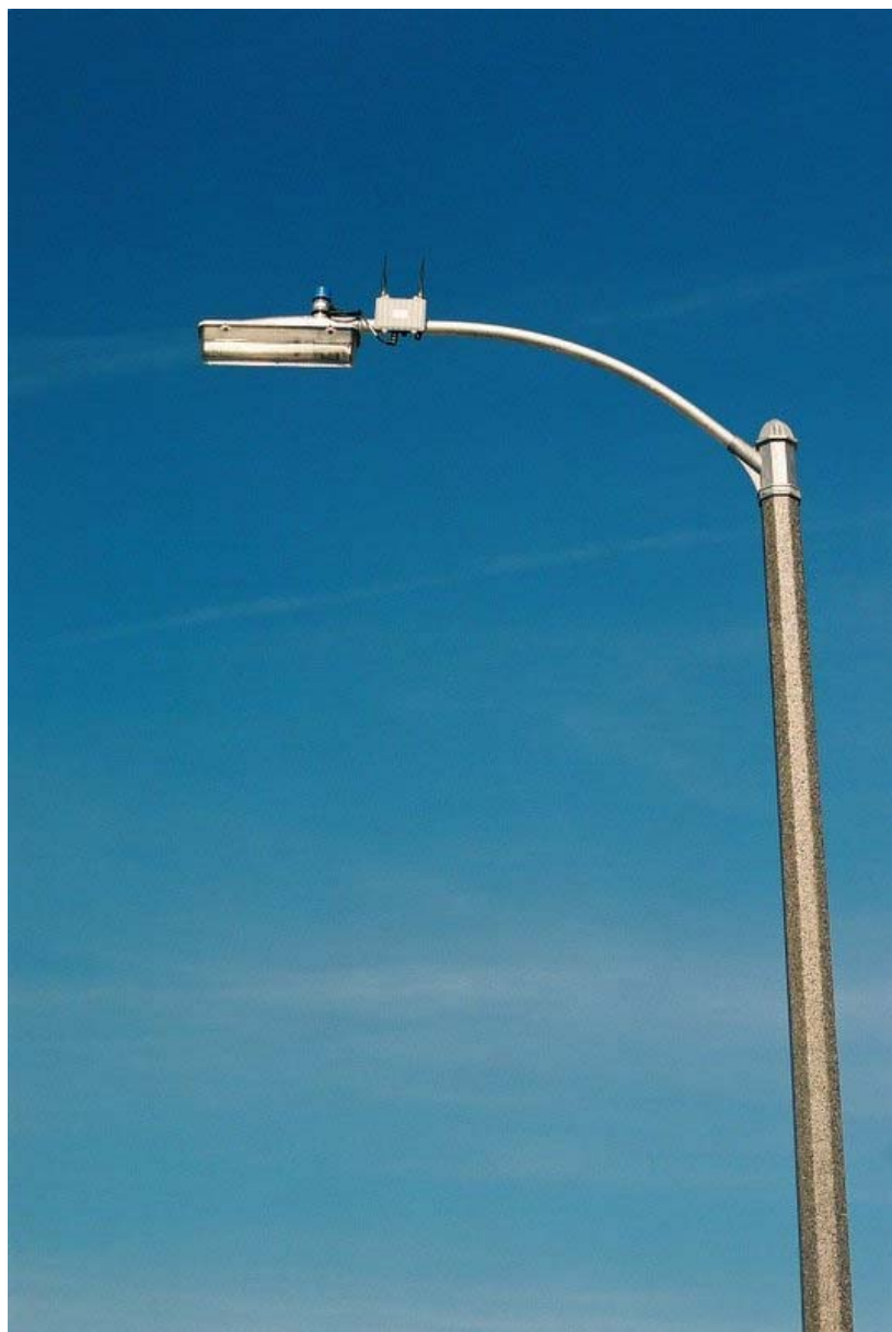
Figure 11. Pole Mount bracket streetlight assembly
