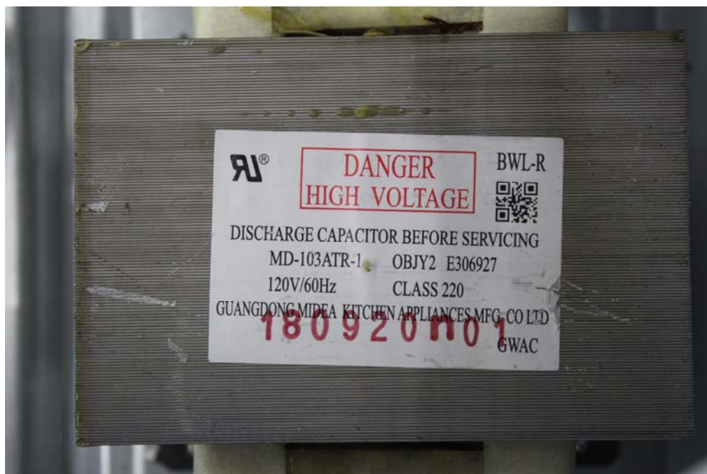
EUT –Transformer View
