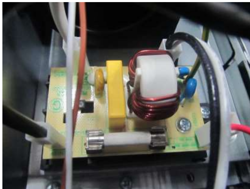
Power Filter Board -Top View
