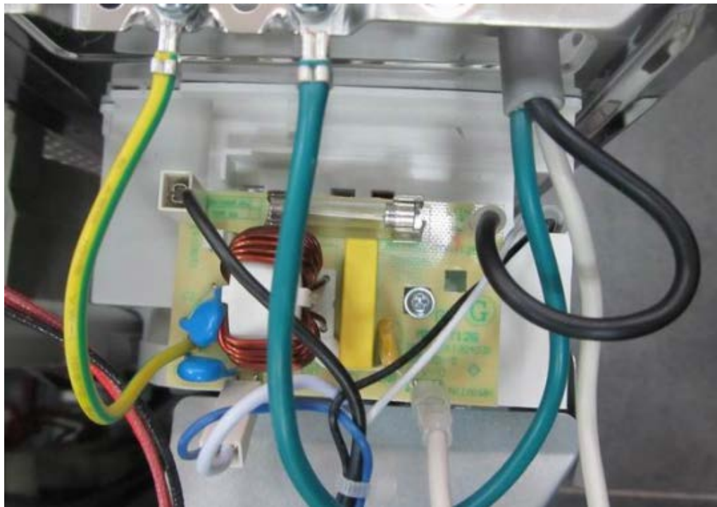
Power Filter Board Top View
