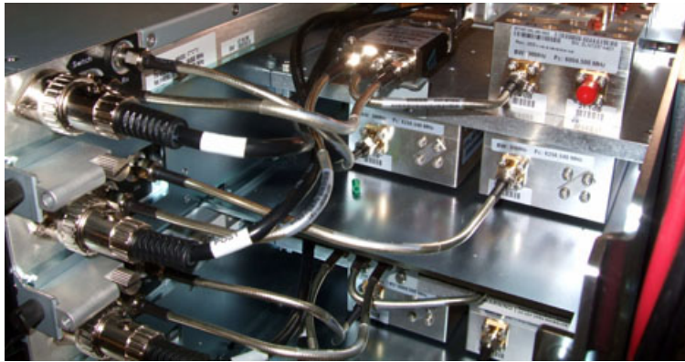
Figure 39. IRU 600v3/v4 Tx Switch and RFUv3 Connections
