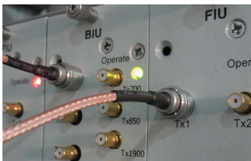
Figure 21 BTS QMA Coaxial Cable Connection
