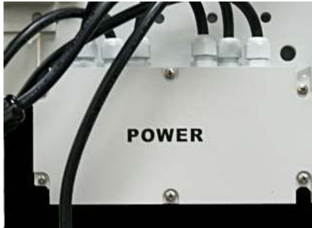
Figure 35 AC Power Junction Box
