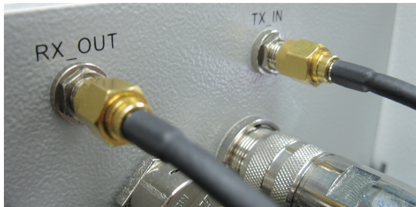
SMA Coaxial Cable Inter-connection on Single-band Enclosure
