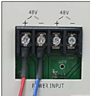
Figure 27 48VDC Host Power Connection
