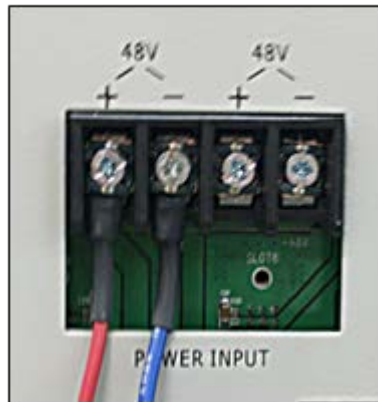
Figure 27 48VDC Host Power Connection
