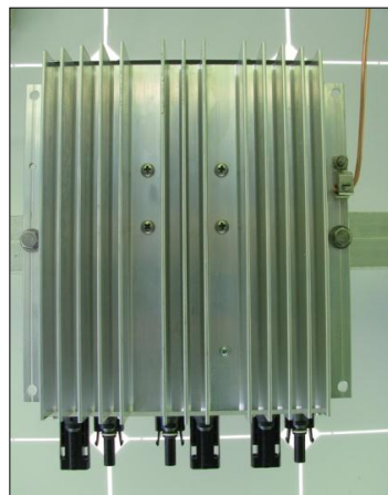
Figure 11: Ampt String Optimizer mounted and grounded
