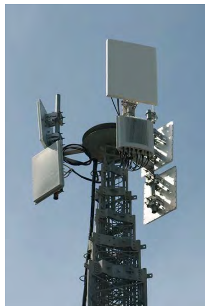
Figure 1 Mercury Quantum 6600 Base Station Mounted on Tower
