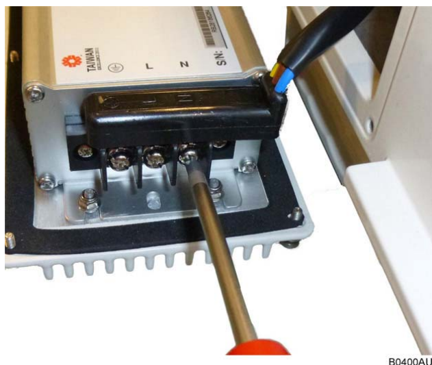
Figure 2-28 RU power supply input cable
