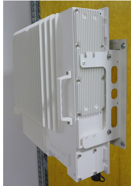
Completed RU Mount
