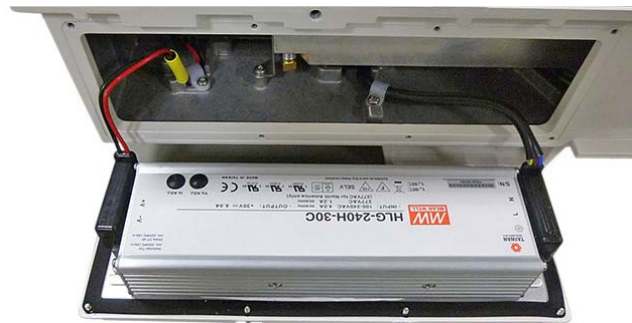
figure 5-4 EU power supply with cables
