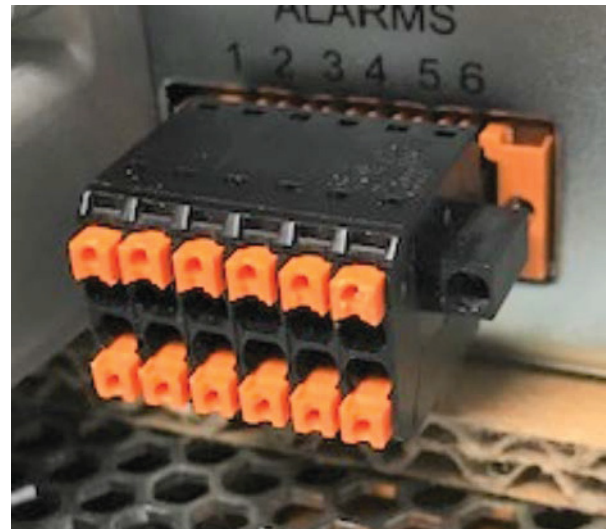
Mating connector inserted into WCS alarm port
