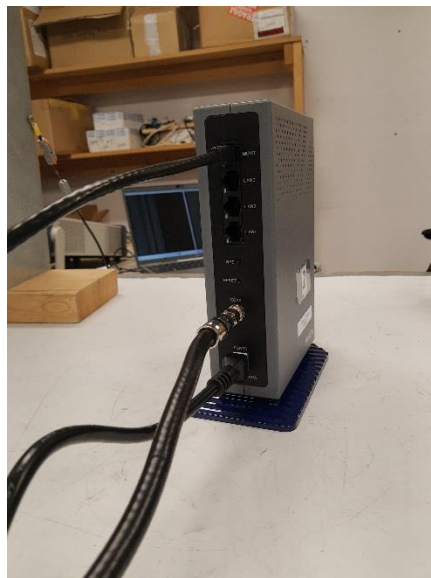
Photograph 4. CNX-WiFi, Rear Side
