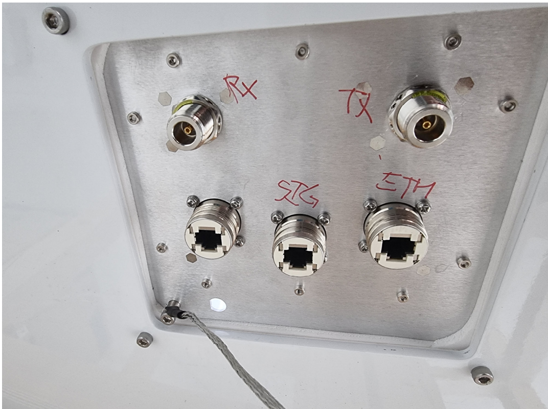
Secondary Antenna (located at Bottom of Antenna)
