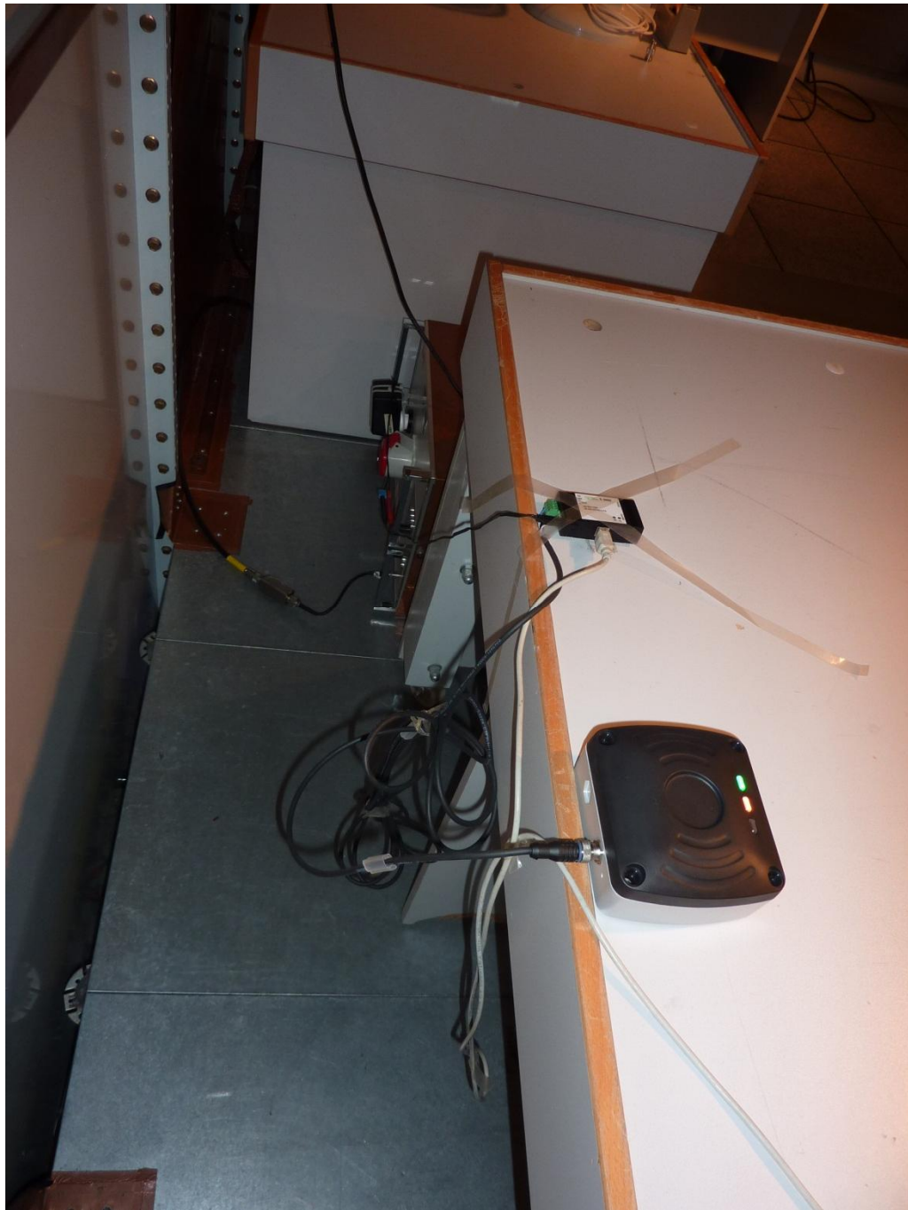
142568_i.JPG: TN902-Q120L130-H1147, test shielded chamber
