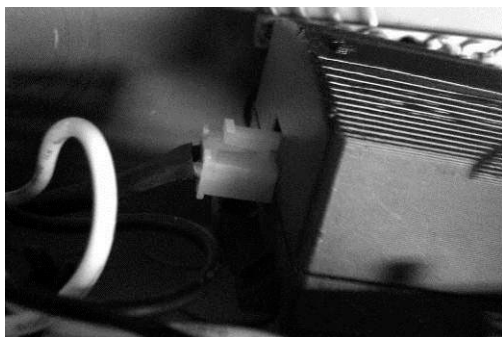
Power Cable attached to ePod
