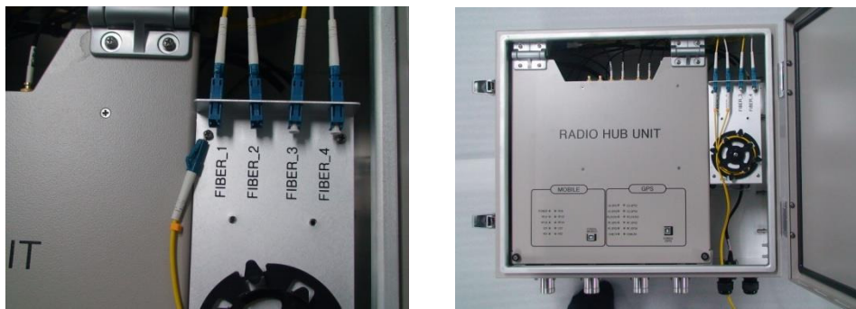
Figure 3-9 Fiber cable connection on RHU
