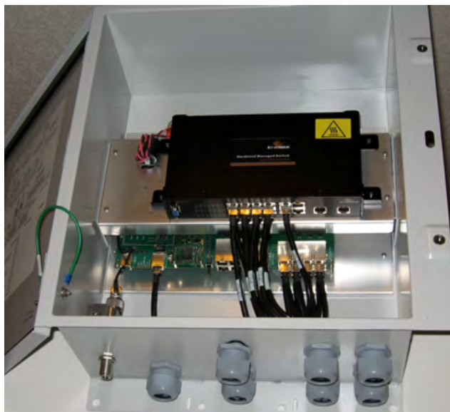
Figure 57: CMM4 (Cabinet with switch)
