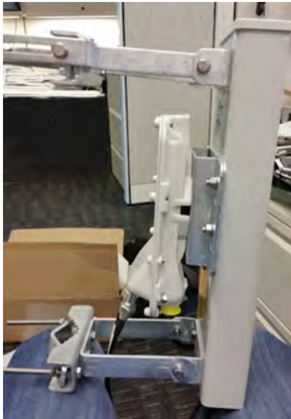
Figure 128: Completed AP and antenna assembly
