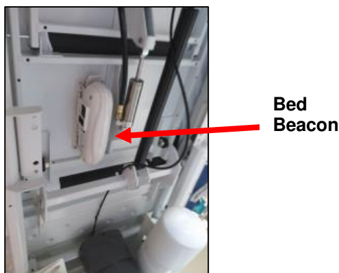
Figure 1. Bed Beacon Installation Location on the Bed
